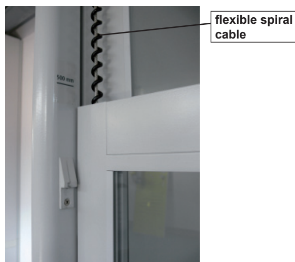
Light barrier cable (flexible spiral cable) twisted around sash wire
